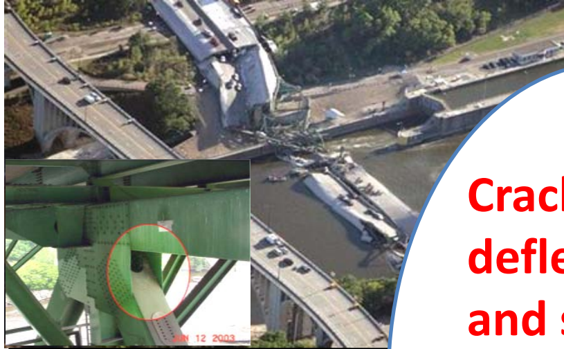
I-25W bridge (US) collapse corrosion of joints
