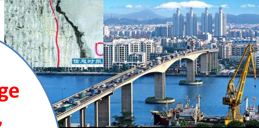
girder bridge' s severe such as Luoxi bridge, safety problems
