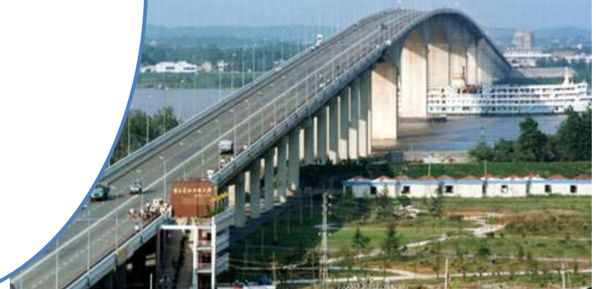
Deflection of girder bridge, such as Huangshi bridge, deflected 33cm after 15 years
